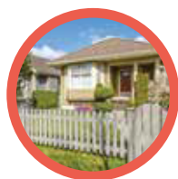
Combustible Wooden Slat Fence
